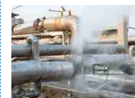
Flue Gas Desulfurization
